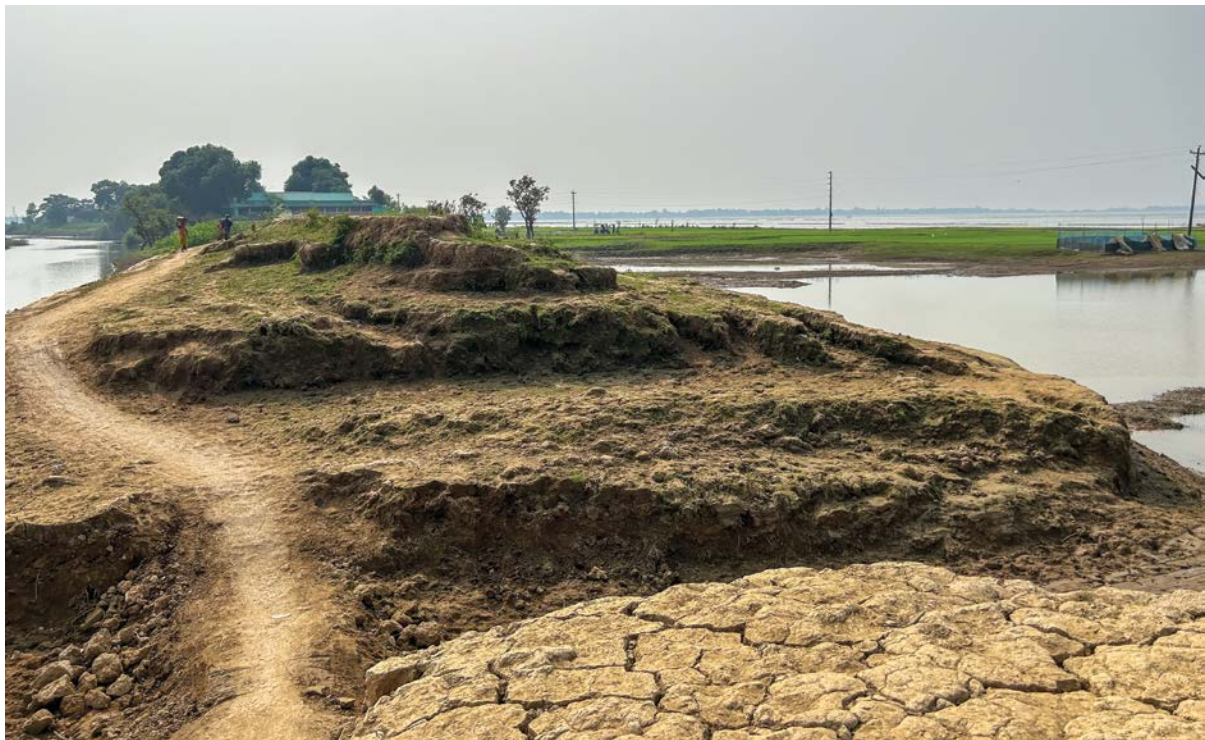
Intense floods break through embankments, cutting off vital roads and exacerbating flooding.
