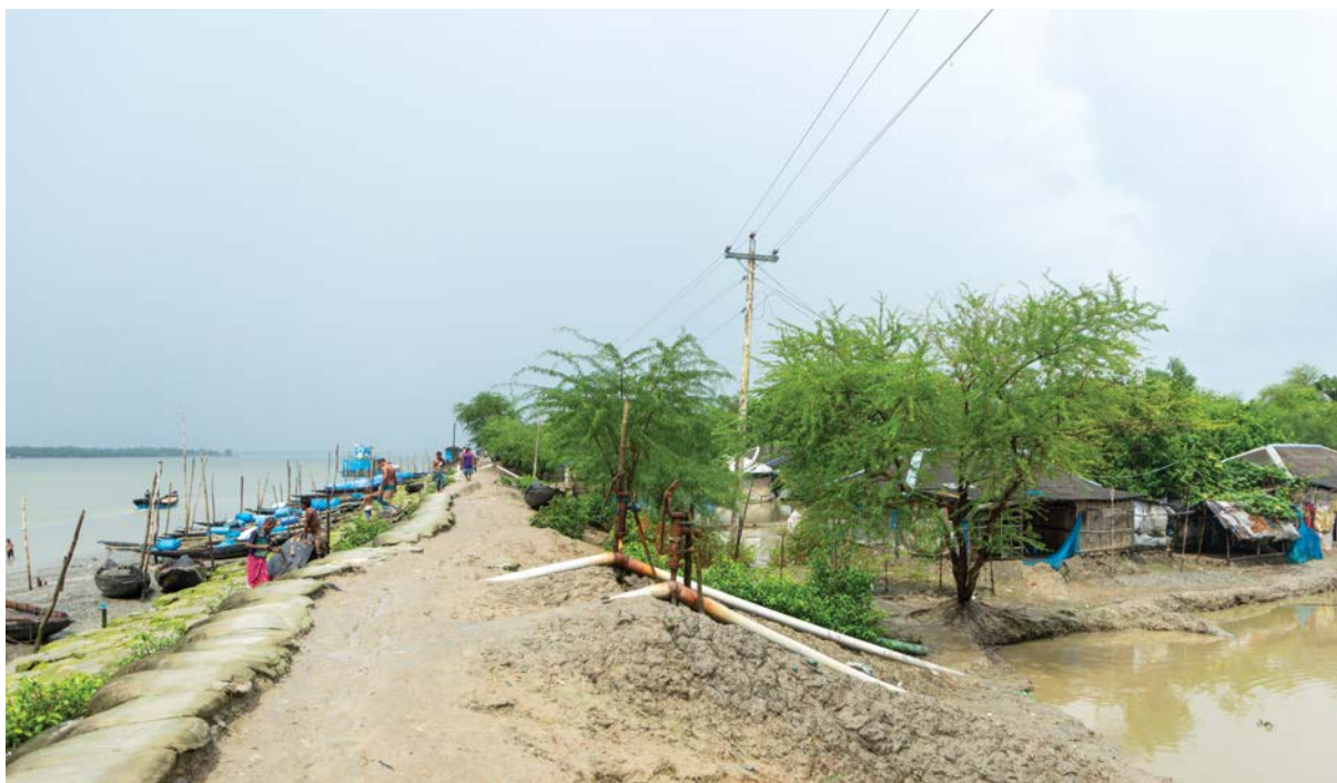
Illegal water channel ("switch gate") diverting saline river water into shrimp farms, contributing to the spread of salinity in nearby agricultural land.
