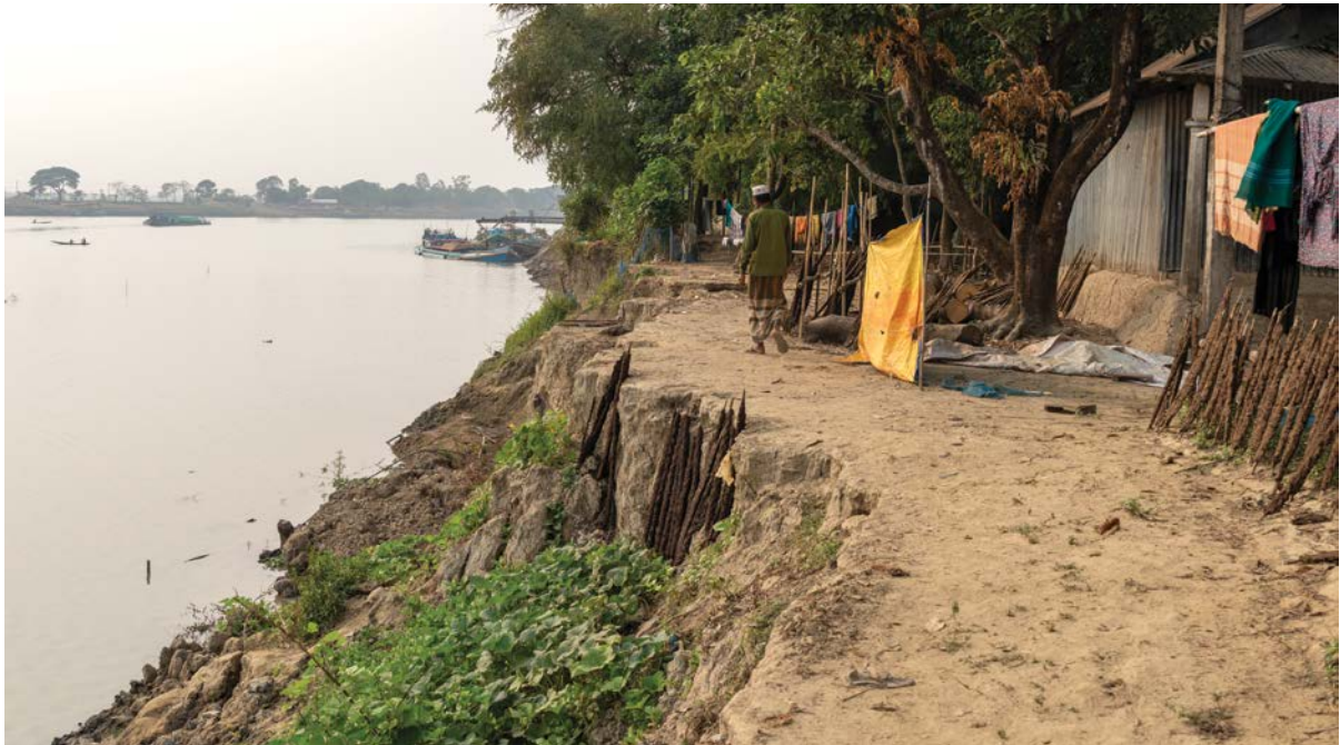
River erosion along the Kushiya and Surma River deepens, driven by climate change and reckless, unplanned development that ignores environmental safeguards.
